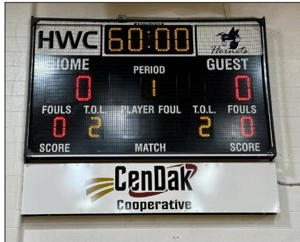
The new scoreboard in the Fessenden-Bowdon School gymnasium was installed last month.
